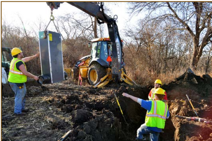
Bioreactor being installed in Polk County, Iowa, by City of Des Moines employees. The bioreactor was designed by the USDA Natural Resources Conservation Service. SWCS/IDALS Photo by Lynn Betts.
