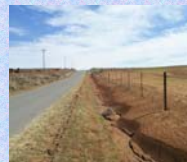
Fig 5. Erosion from roadside ditch.
